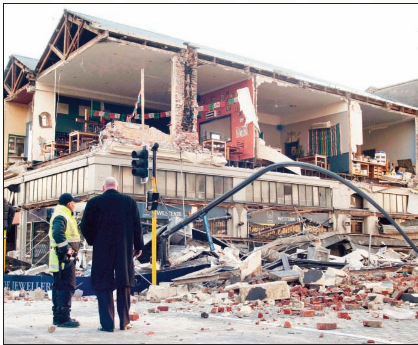
AP PHOTO People stand outside a building damaged by a 7.4-magnitude earthquake in central Christchurch, New Zealand early today. There were no reports of injuries, but looters broke into some damaged shops in Christchurch, police said.
